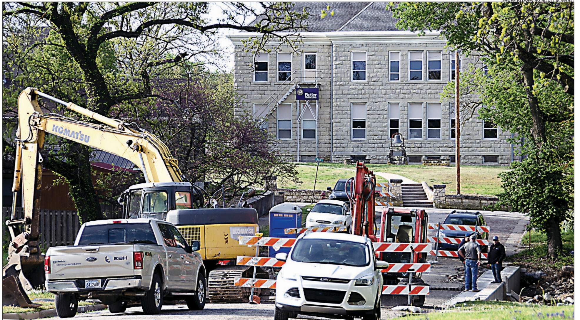
Workers are nearly finished with a long-delayed repair of Marion's Locust St. north of Main St. Erosion had left as much as eight feet of a box bridge under the street hanging in the air and endangered a retaining wall at the edge of the street. The state awarded a grant that would pay 70% of the $290,727 cost of repairs, plus new curbing from Lawrence to Main Sts. in October, 2022. Work began two weeks ago. Elm St. will be closed next week to excavate existing drainage pipes beneath the street and replace it with new pipes. Curbing also will be replaced. The same 70% grant for the Locust St. work includes the Elm St. work.
