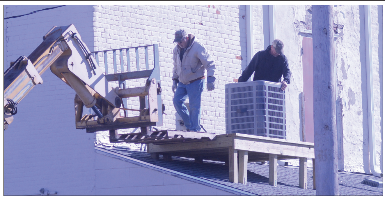
Roger Demanette and Galen LaBarge installing two AC units for the American Legion in downtown Concordia, with the help of a crane operated by Greg Peltier of Peltier Steel & Fabrication.
